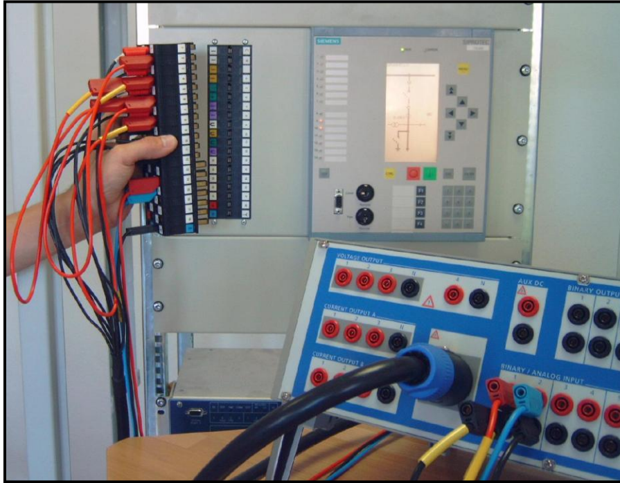
Image 1: Protective Relay, Test Block and Test Plug with a Test Set
